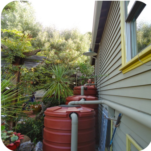
Daisy chained system of 205-gallon rain barrels Courtesy of The City of Oakland
