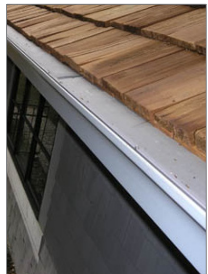
This gutter is covered by a fine mesh gutter guard to keep debris out.
