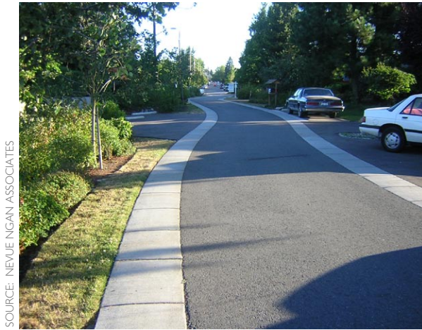
Figure 5-26: This “curbless” street example allows for sheet flow of runoff into a vegetated swale.
